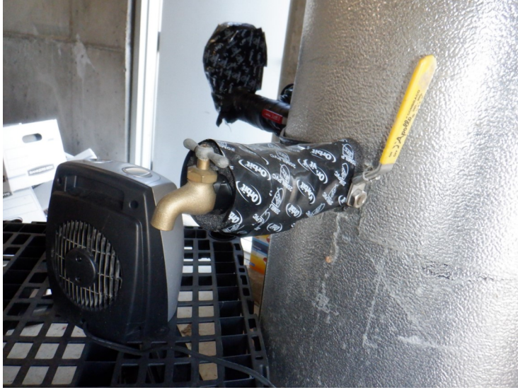
31) The sample tap on the fill/draw pipe is in good condition.
