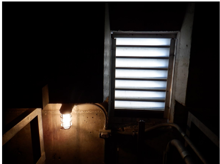
38) The louvered vent at the top of the column is in good condition.
