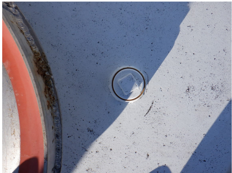
17) The roof rigging couplings are capped.
