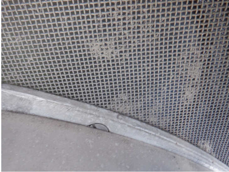
25) The roof vent screened pressure plate is was found to be properly aligned.
