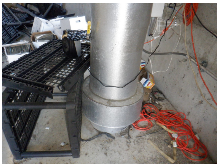
30) The expansion joint at the bottom of the fill/draw pipe is covered with insulation and not accessible for inspection.
