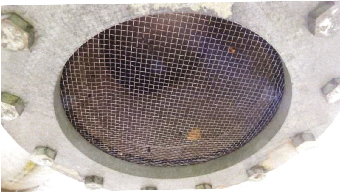
Photos show the 12" overflow pipe system, which is not equipped with a flapper valve as required by AWWA D107-16; 8.7.5 Overflow piping . We recommend installing a flapper valve and new screen on the existing overflow pipe elbow.
