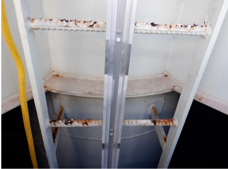
58) There is minor steel loss from corrosion on the top three ladder rungs in the wet interior.
