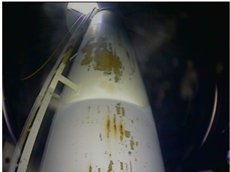
56) The access tube coating is in poor condition with multiple failures.
