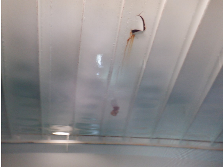
46) There are coating failures on the wet interior roof.
