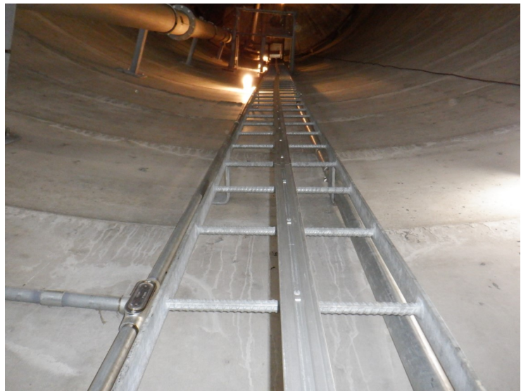
32) The dry interior ladder is in good condition. The ladder is equipped with a fall prevention device.
