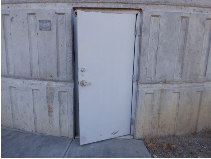
1) The column service door operated properly.
