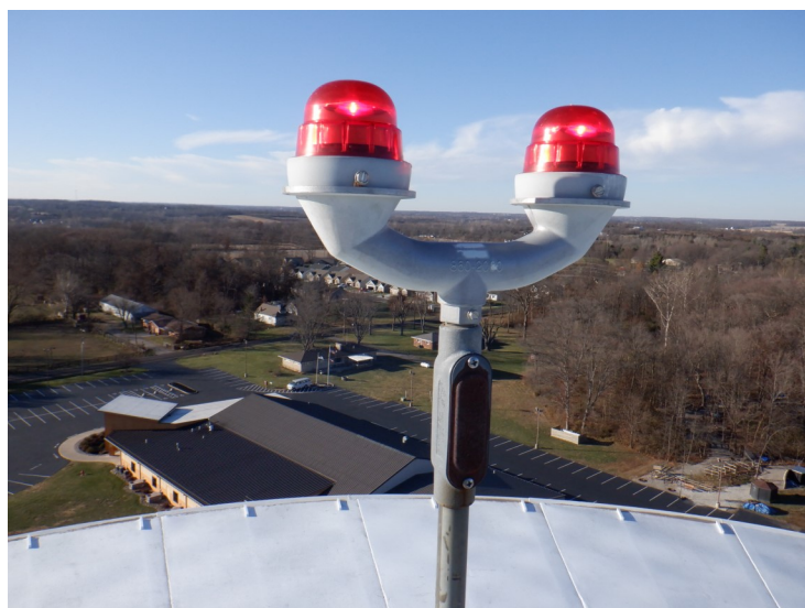
27) The double aviation light is functioning.
