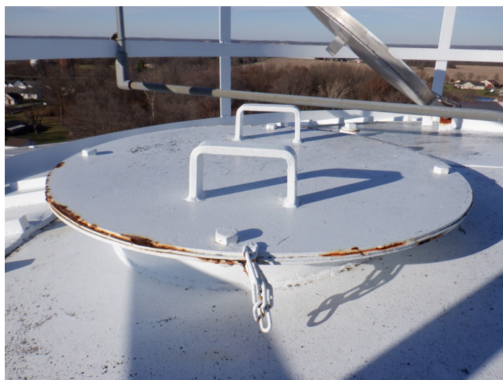
21) There is corrosion at the edges of the bolted ventilation hatch.
