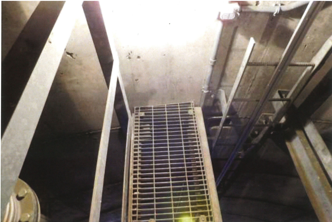
Photo shows the transfer walkway, from the access ladder to the access tube, which is equipped with 42" high OSHA compliant handrail system, and appears to be in good condition.
