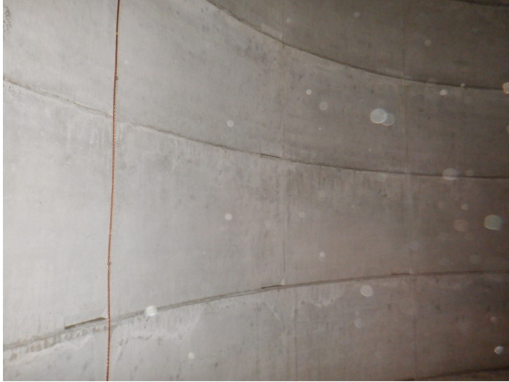
28) The concrete column in the dry interior is in good condition with no deterioration.
