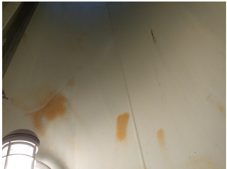
41) There are a few areas of rust bleedthrough in the access tube.
