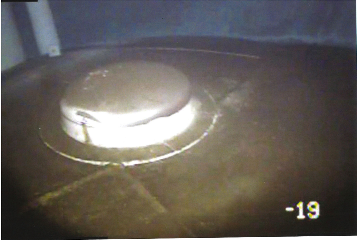
Photo shows the tank floor manhole, which is in compliance with AWWA D107-16; 8.4.5 Tank floor manhole and appears to be in good condition.
