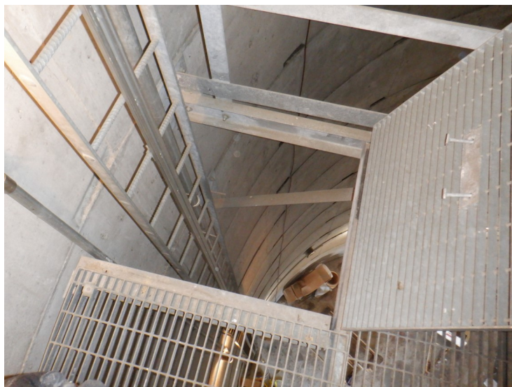
33) The ladder openings at the interior platforms are equipped with hinged covers.
