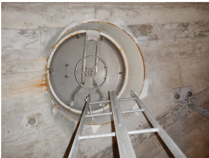
36) The wet interior manway in the domed bottom is in good condition.
