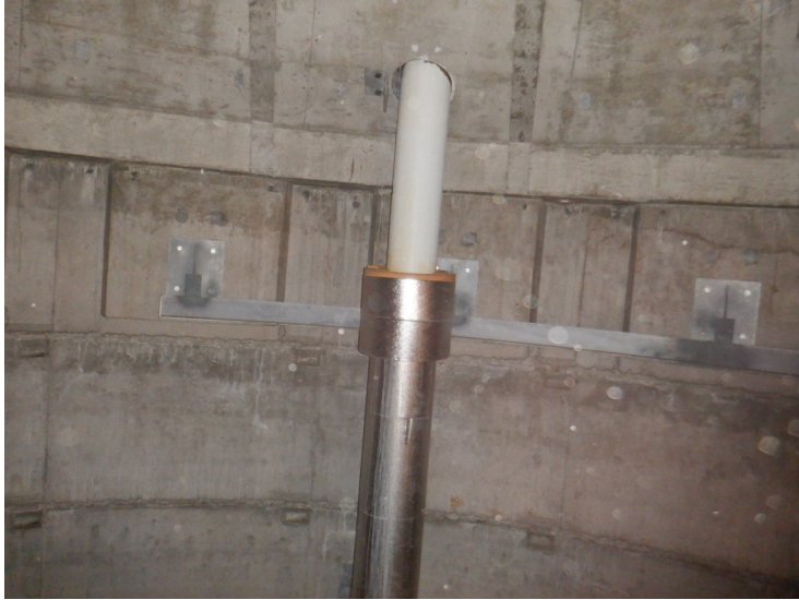
34) The fill/draw pipe insulation and aluminum jacket are in good condition. The painter's railing at the top of the column is in good condition.
