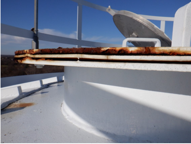
22) There is a gasket on the bolted ventilation hatch.
