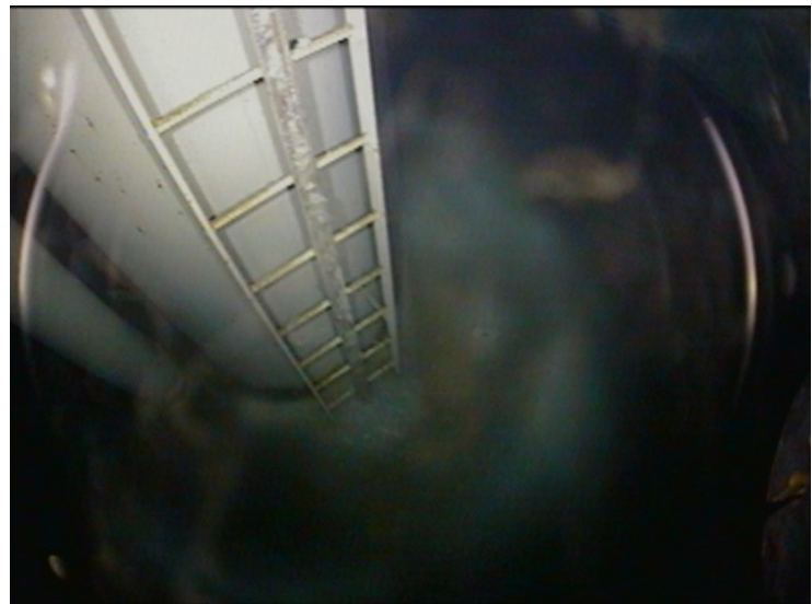
59) The wet interior ladder appears to be in good condition. The ladder is equipped with a fall prevention device.
