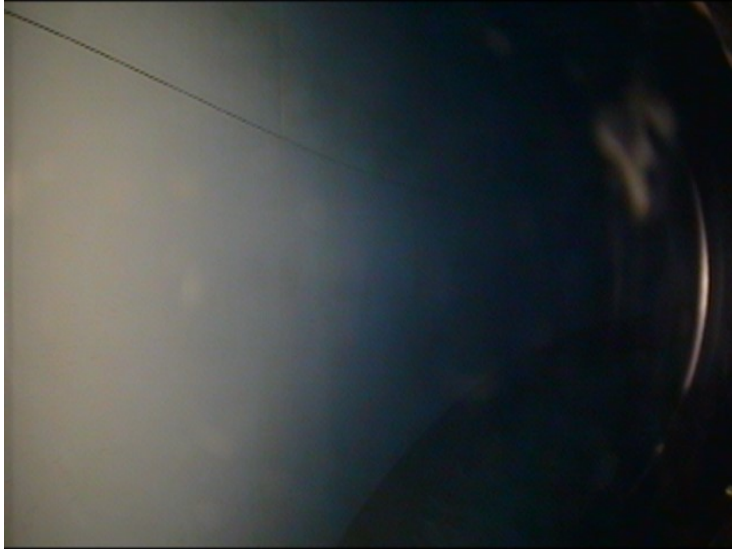
55) The wet interior sidewall coating is in fair condition overall.
