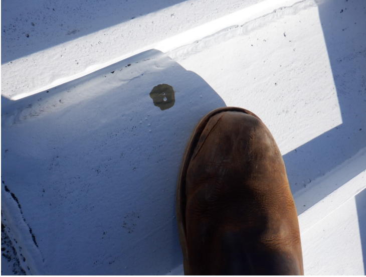
13) There are a few minor coating failures on the roof.
