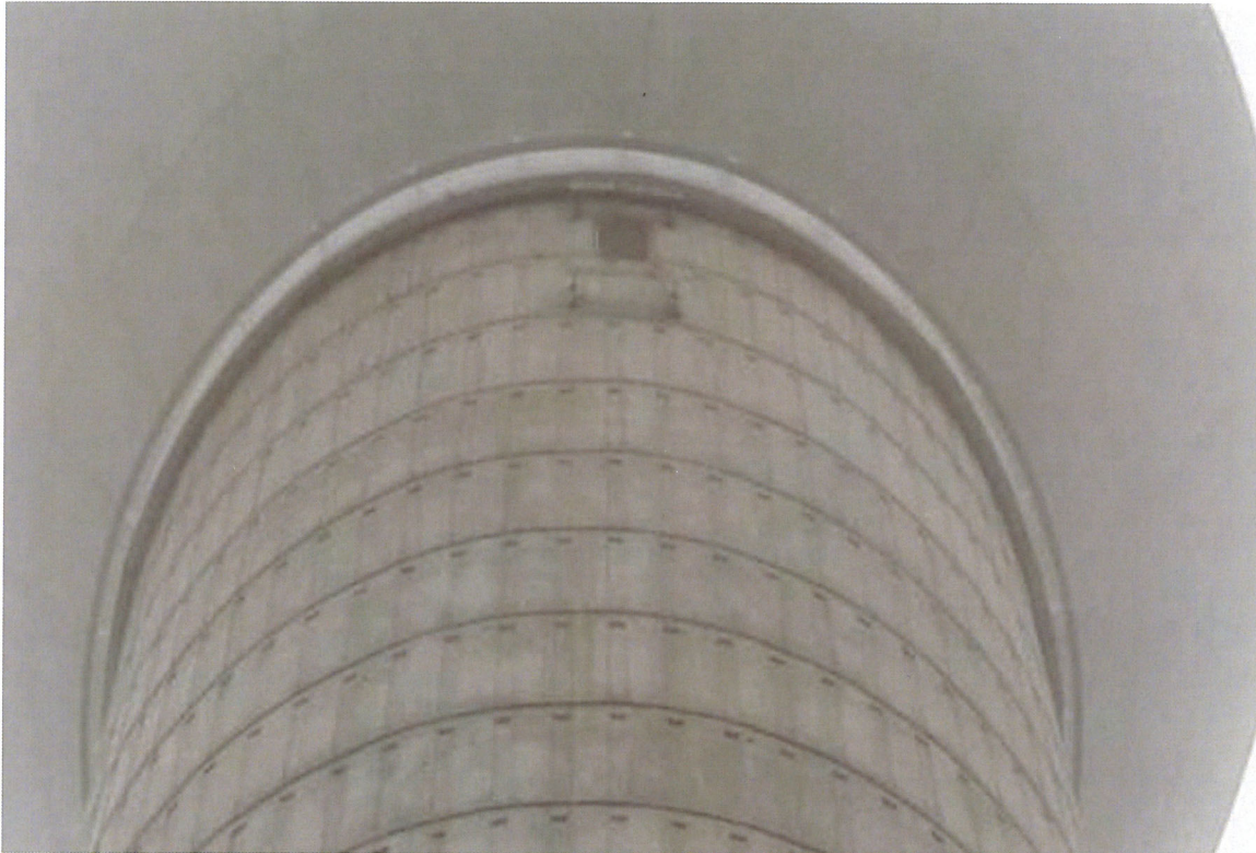
Photo shows one of the pedestal vents, which appears to be in good condition.
