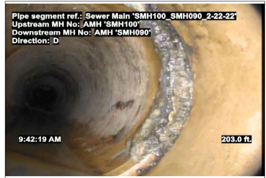
At: 203 ft. 2/5 DAE - Deposits Attached Encrustation Joint: No 5 %
