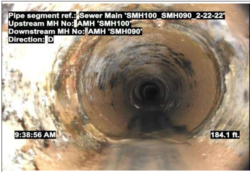
At: 184.1 ft. 7/1 DAE - Deposits Attached Encrustation Joint: No 5%
