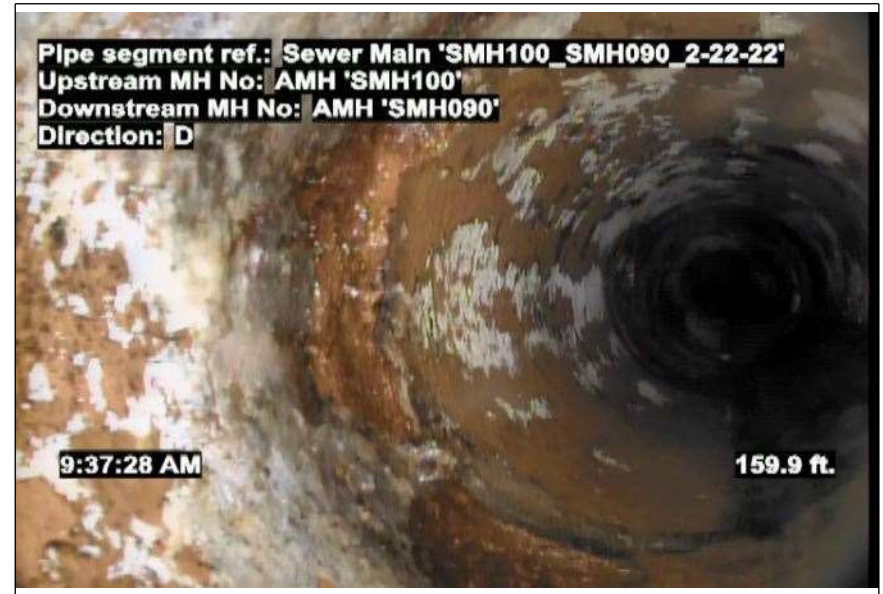
At: 159.9 ft. 7/10 DAE - Deposits Attached Encrustation Joint: No 5%
