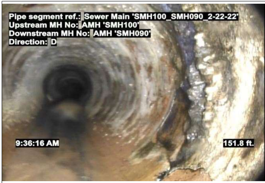
At: 151.8 ft. 1/4 DAE - Deposits Attached Encrustation Joint: No 5%
