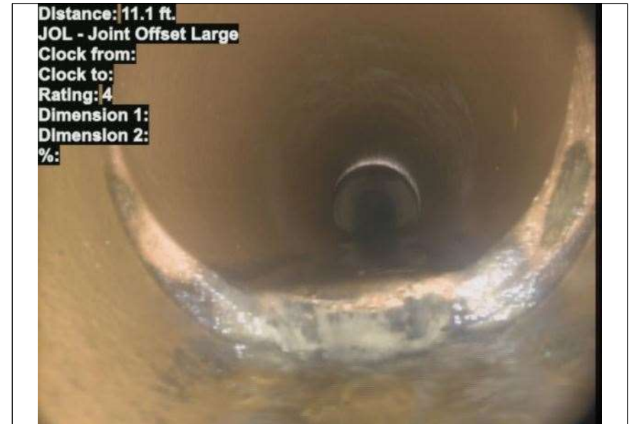
At: 11.1 ft. JOL - Joint Offset Large Joint: No
