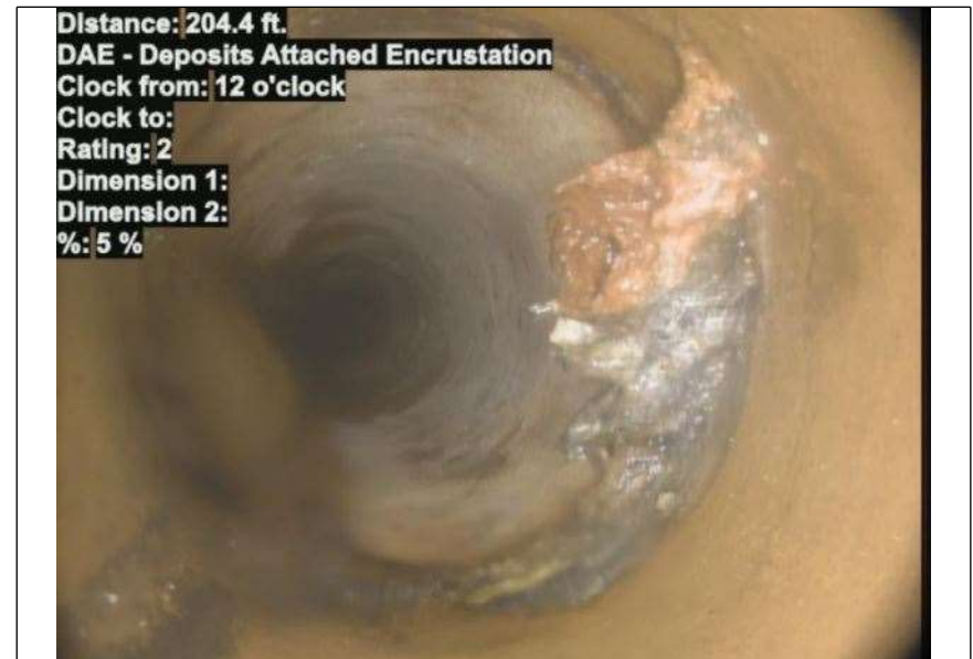
At: 204.4 ft. 12/. DAE - Deposits Attached Encrustation Joint: No 5 %
