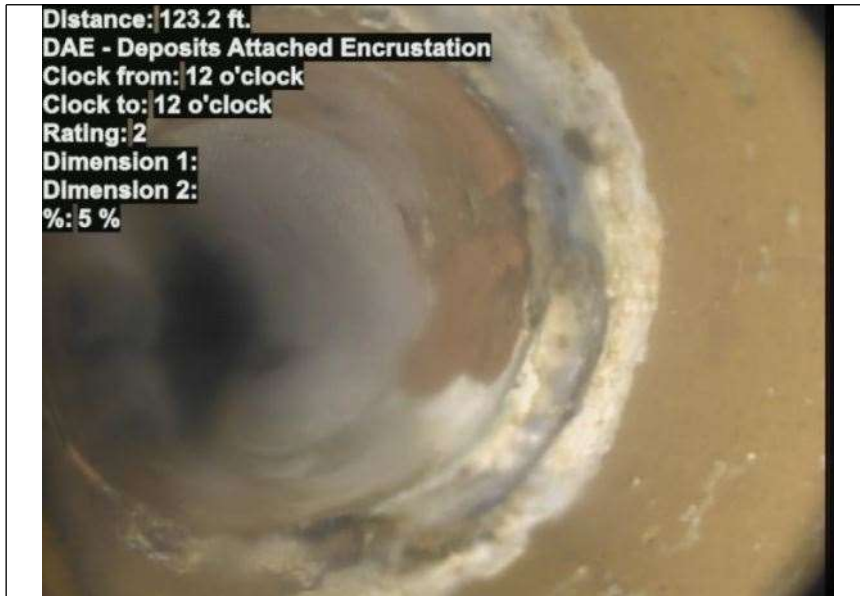
At: 123.2 ft. 7/5 DAE - Deposits Attached Encrustation Joint: No 5 %
