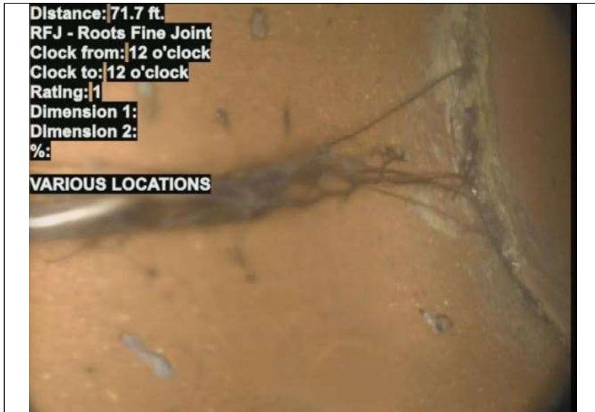
At: 71.7 ft. 7/5 RFJ - Roots Fine Joint Joint: Yes VARIOUS LOCATIONS
