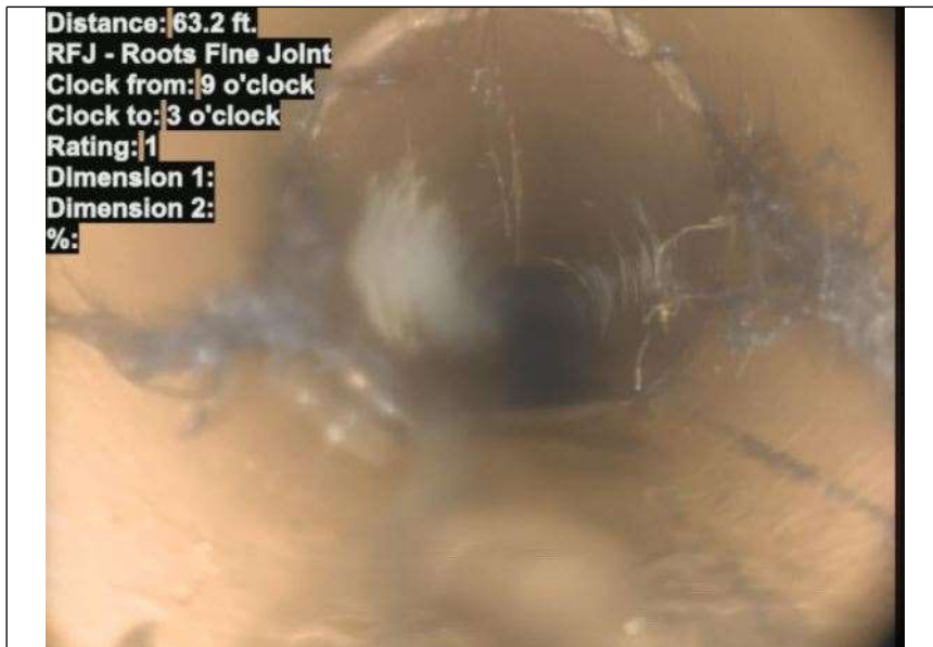
At: 63.2 ft. 9/3 RFJ - Roots Fine Joint Joint: Yes
