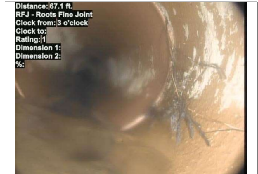
At: 67.1 ft. 3/ RFJ - Roots Fine Joint Joint: Yes
