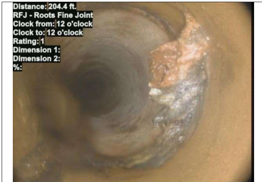
At: 204.4 ft. 7/5 RFJ - Roots Fine Joint Joint: Yes
