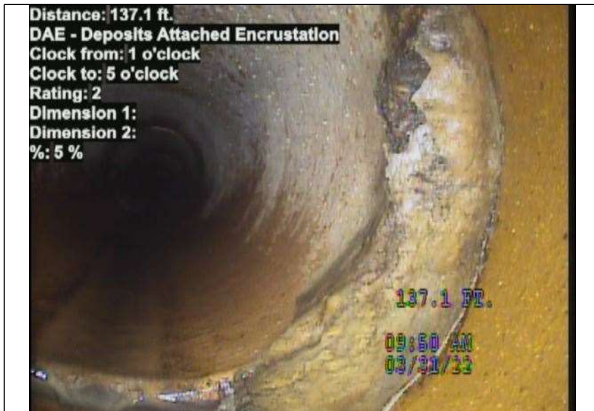
At: 137.1 ft. 1/5 DAE - Deposits Attached Encrustation Joint: No 5 %
