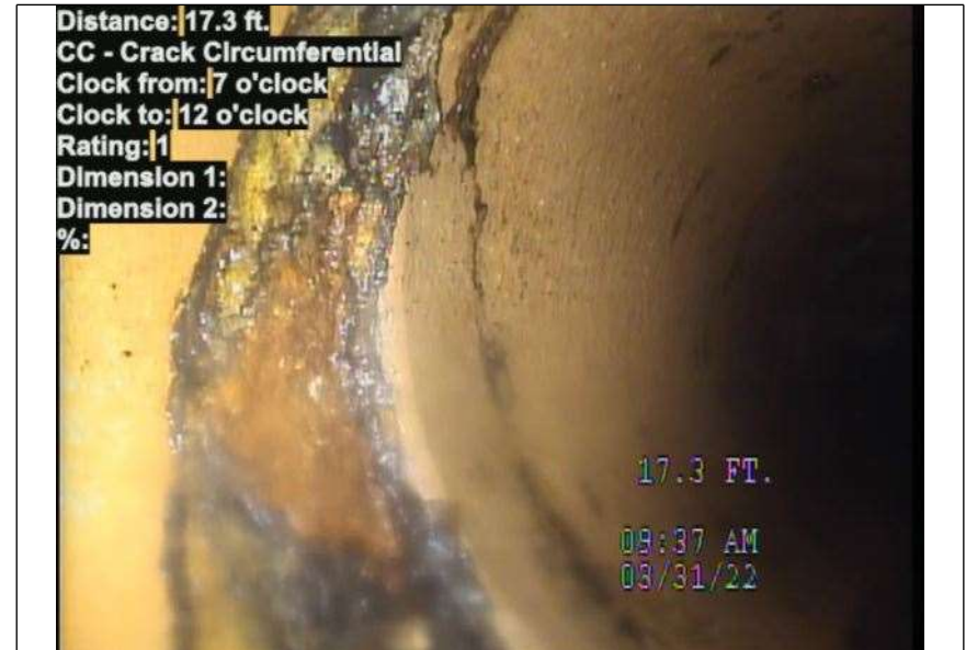
At: 17.3 ft. 7/12 CC - Crack Circumferential Joint: No
