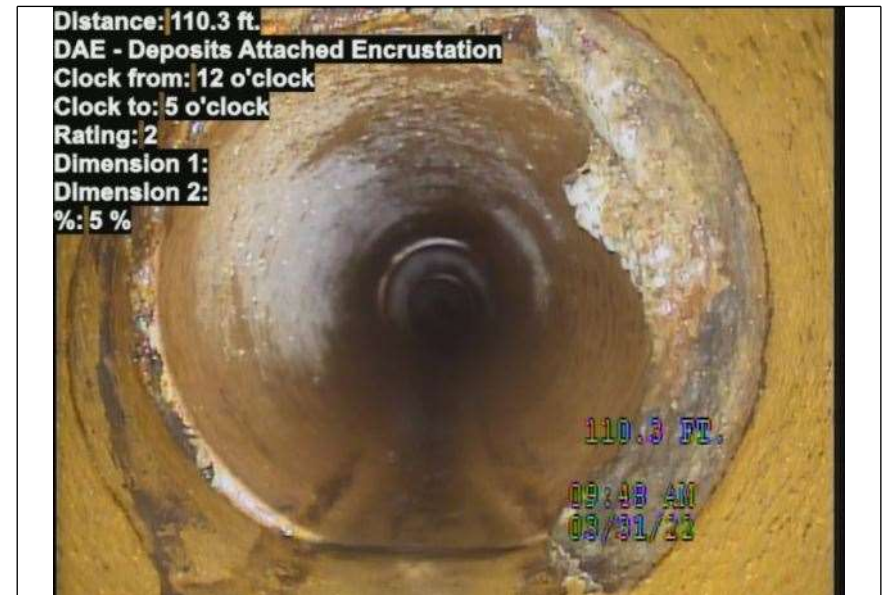
At: 110.3 ft. 12/5 DAE - Deposits Attached Encrustation Joint: No 5 %
