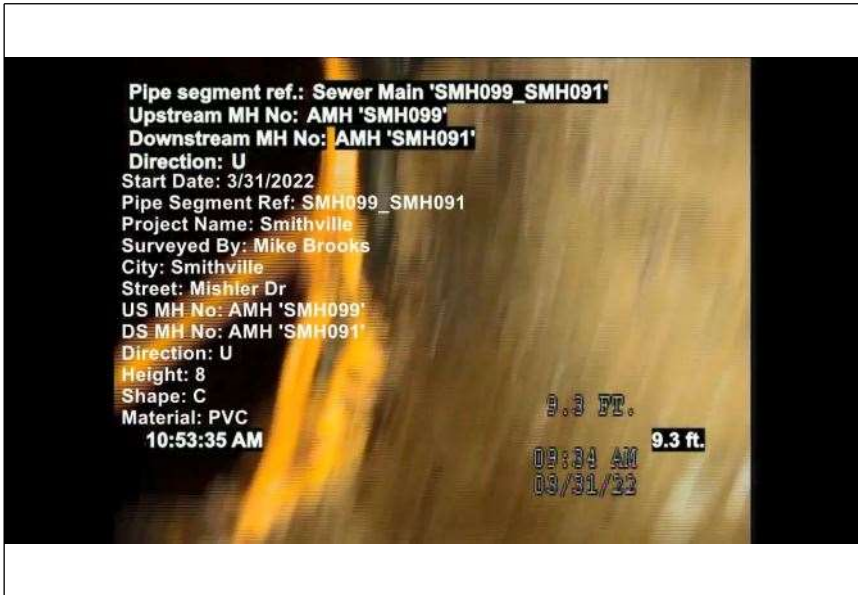
At: 0 ft. AMH - Manhole Joint: No SMH091
