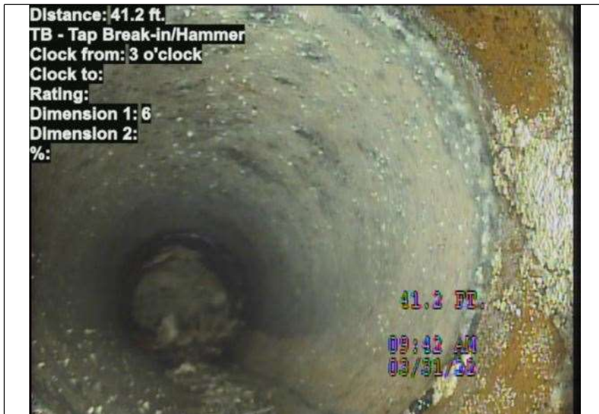
At: 41.2 ft. 3/. TB - Tap Break-in/Hammer Joint: No
