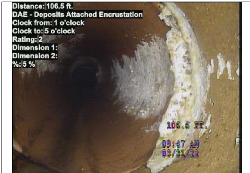
At: 106.5 ft. 1/5 DAE - Deposits Attached Encrustation Joint: No 5 %
