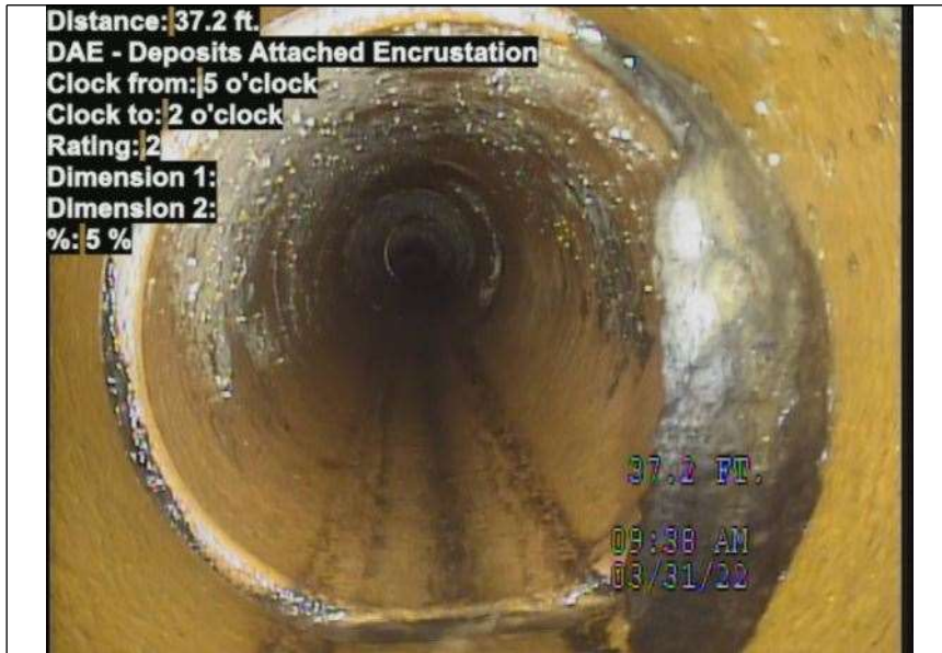
At: 37.2 ft. 5/2 DAE - Deposits Attached Encrustation Joint: No 5 %
