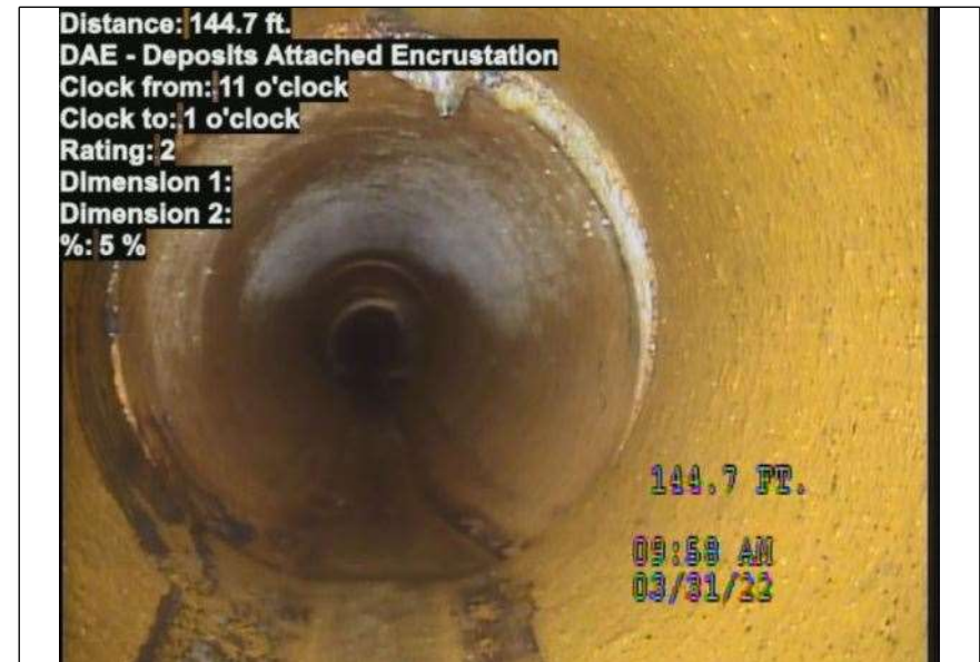
At: 144.7 ft. DAE - Deposits Attached Encrustation 11/1 Joint: No 5 %
