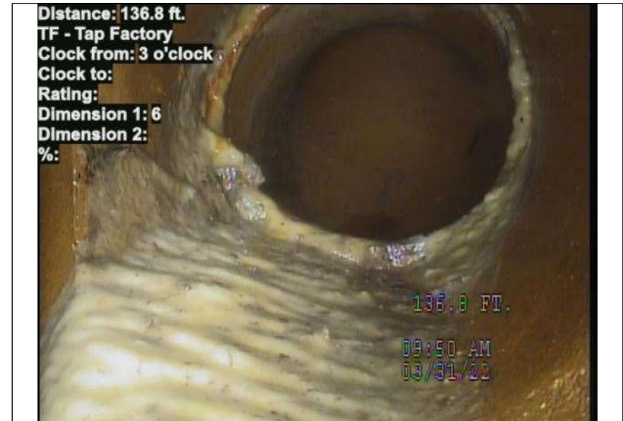
At: 136.8 ft. 3/. TF - Tap Factory Joint: No
