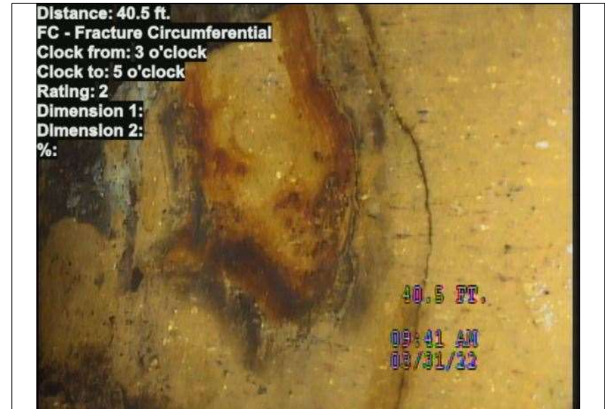
At: 40.5 ft. 3/5 FC - Fracture Circumferential Joint: No
