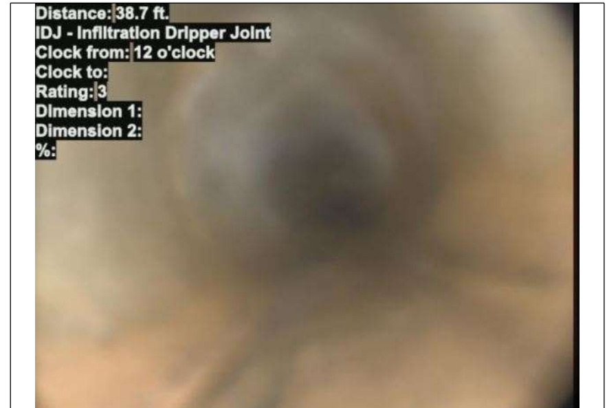
At: 38.7 ft. 12/ IDJ - Infiltration Dripper Joint Joint: Yes
