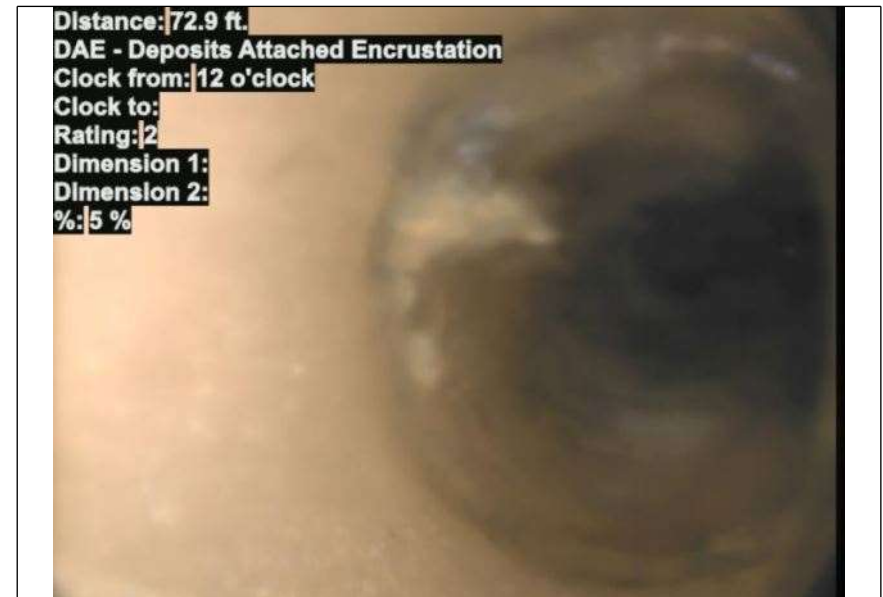
At: 72.9 ft. 12/. DAE - Deposits Attached Encrustation Joint: Yes 5 %
