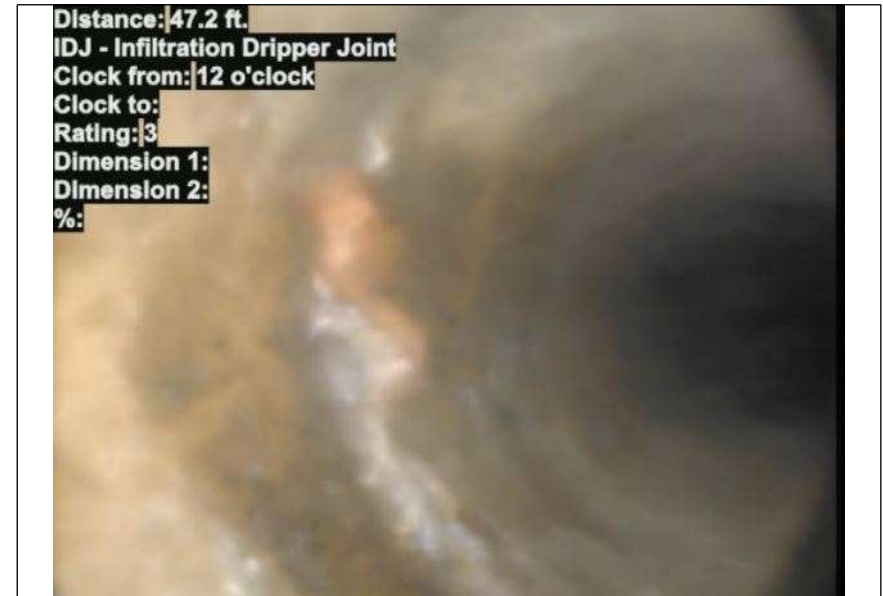
At: 47.2 ft. 12/. IDJ - Infiltration Dripper Joint Joint: Yes
