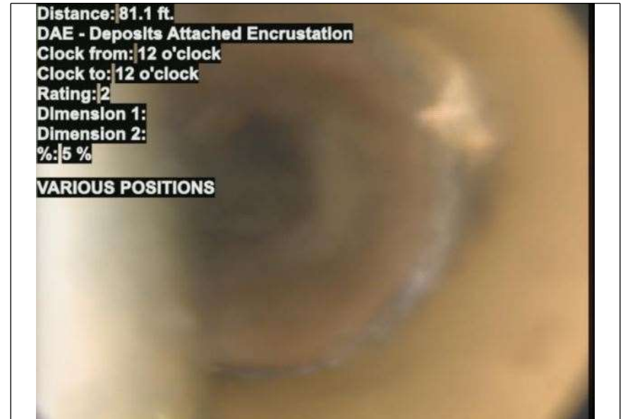
At: 81.1 ft. 7/5 DAE - Deposits Attached Encrustation Joint: Yes 5 % VARIOUS POSITIONS
