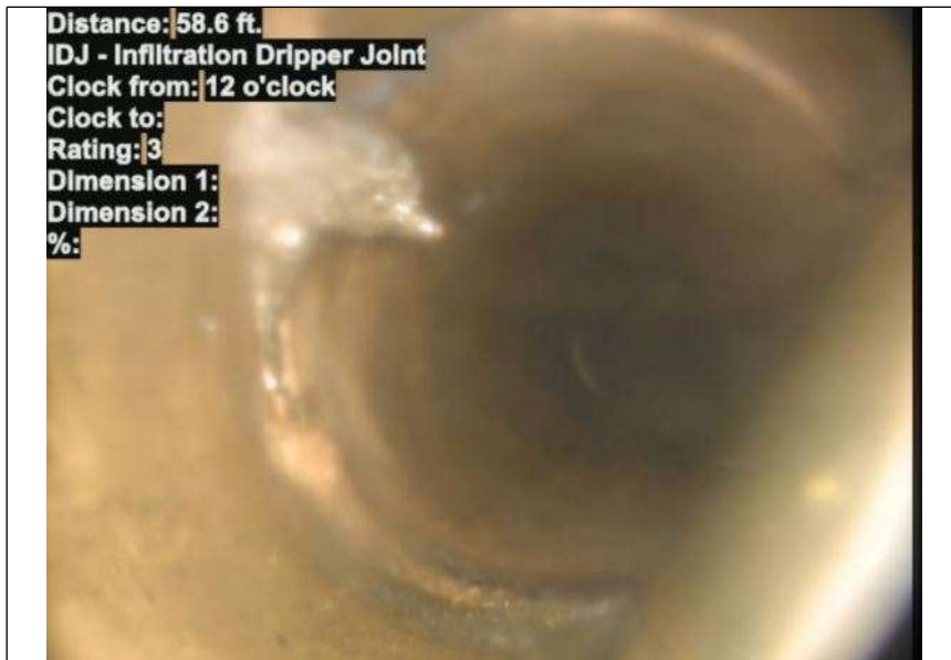
At: 58.6 ft. 12/. IDJ - Infiltration Dripper Joint Joint: Yes
