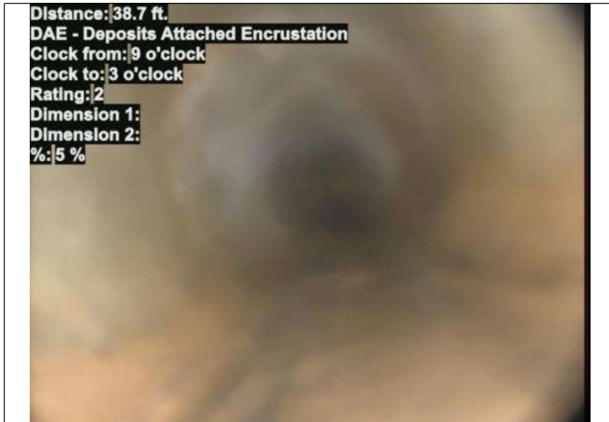
At: 38.7 ft. 9/3 DAE - Deposits Attached Encrustation Joint: Yes 5 %
