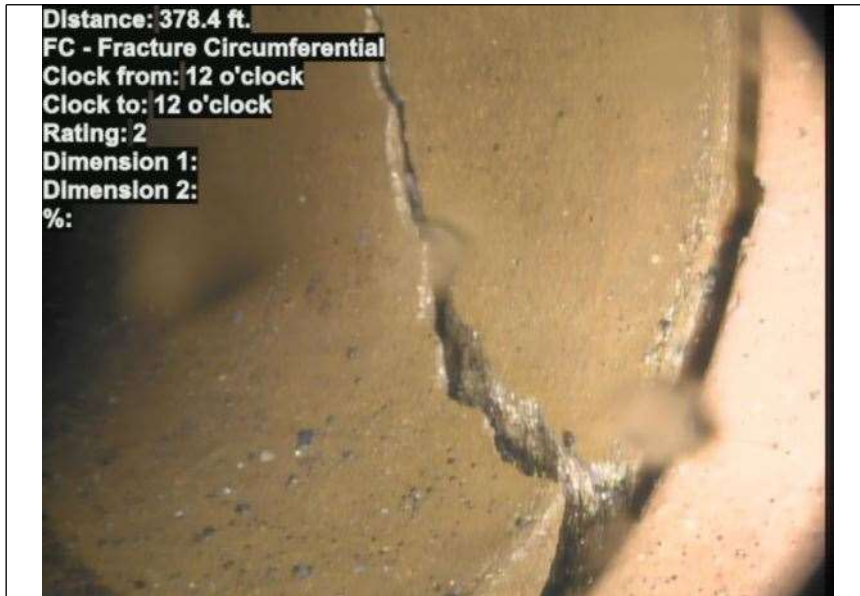
At: 378.4 ft. FC - Fracture Circumferential 12/12
