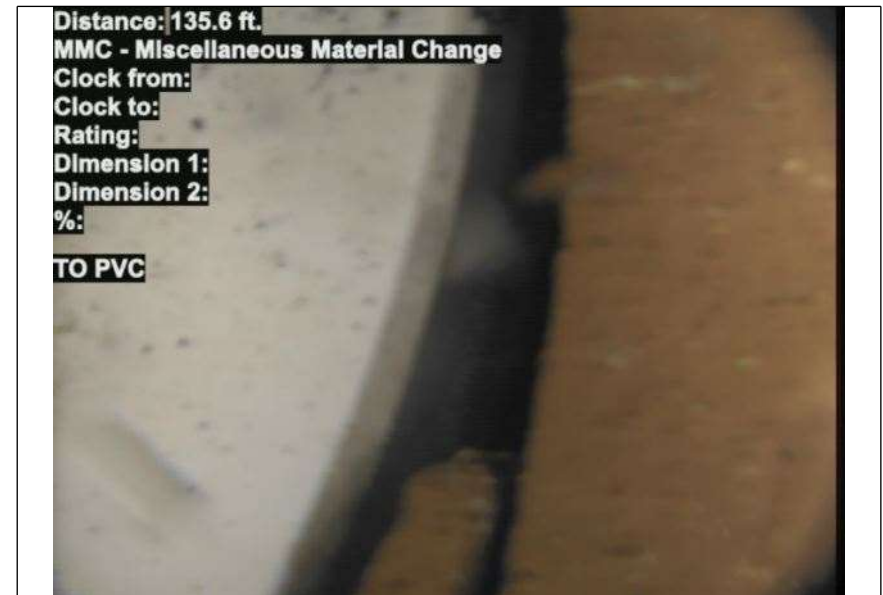
At: 135.6 ft. RPR - Point Repair Replacement Joint: No TO PVC
