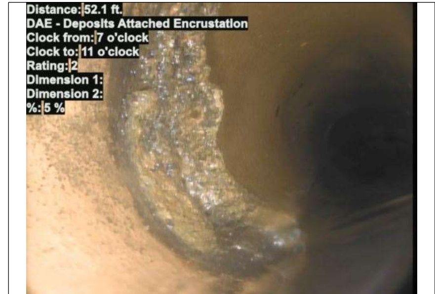
At: 52.1 ft. 7/11 DAE - Deposits Attached Encrustation Joint: No 5 %
