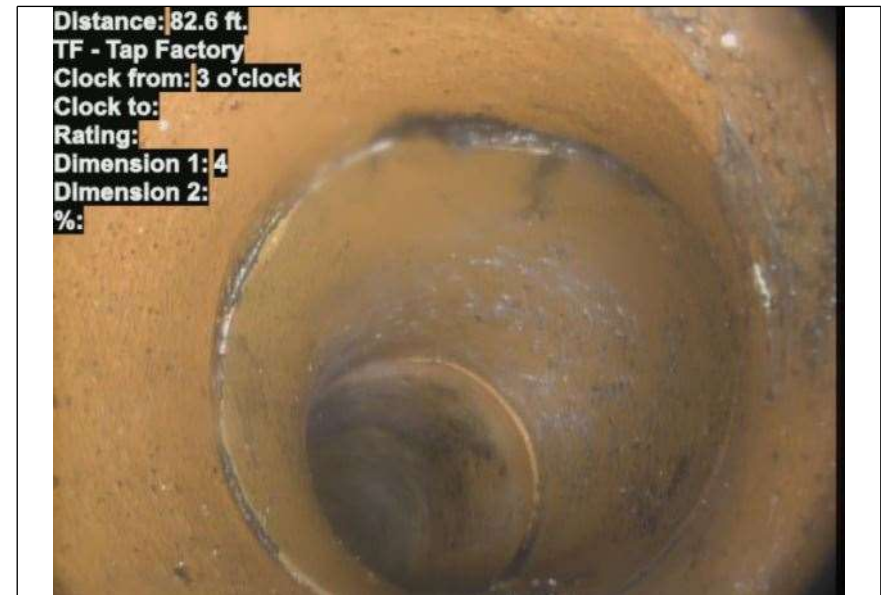
At: 82.6 ft. 3/. TF - Tap Factory Joint: No
