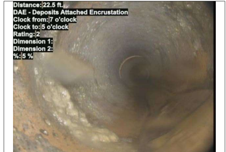
At: 22.5 ft. 7/5 DAE - Deposits Attached Encrustation Joint: Yes 5 %
