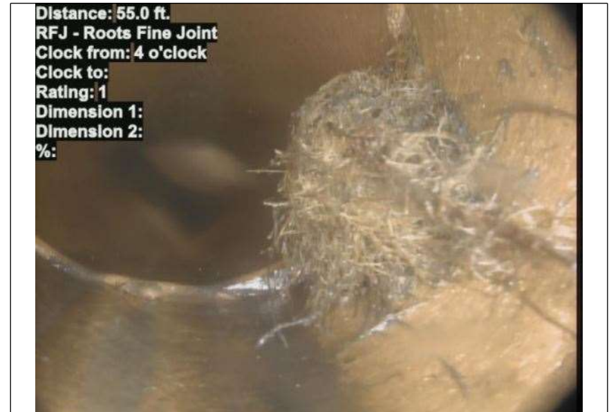
At: 55 ft. 4/. RFJ - Roots Fine Joint Joint: Yes
