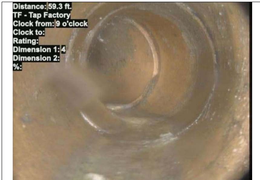
At: 59.3 ft. 9/. TF - Tap Factory Joint: No
