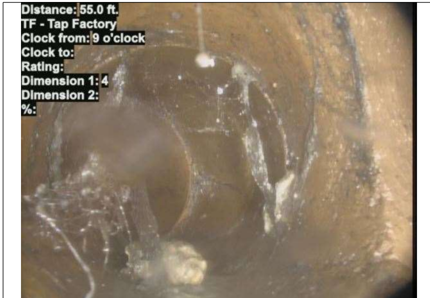
At: 55 ft. 9/. TF - Tap Factory Joint: No
