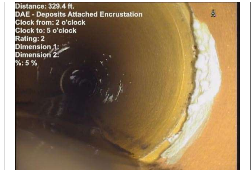
At: 329.4 ft. 2/5 DAE - Deposits Attached Encrustation Joint: No 5 %
