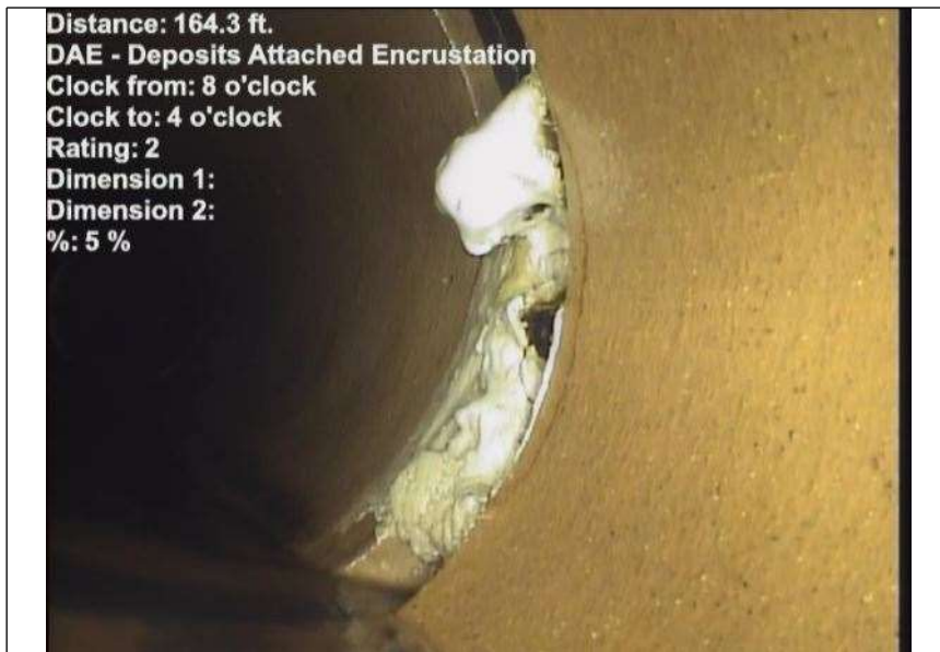
At: 164.3 ft. 8/4 DAE - Deposits Attached Encrustation
