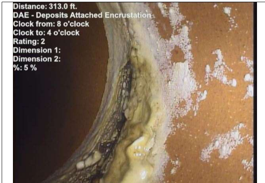
At: 313 ft. 8/4 DAE - Deposits Attached Encrustation Joint: No 5 %
