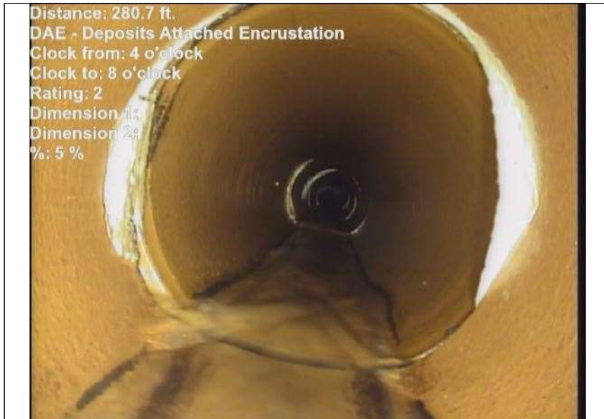
At: 280.7 ft. 4/8 DAE - Deposits Attached Encrustation Joint: No 5 %
