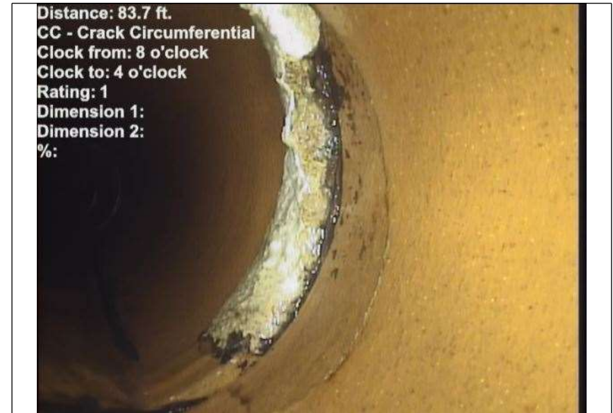
At: 83.7 ft. 8/4 CC - Crack Circumferential Joint: No
