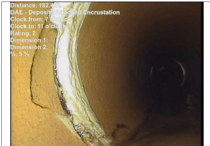
At: 182.4 ft. DAE - Deposits Attached Encrustation 7/11 Joint: No 5 %
