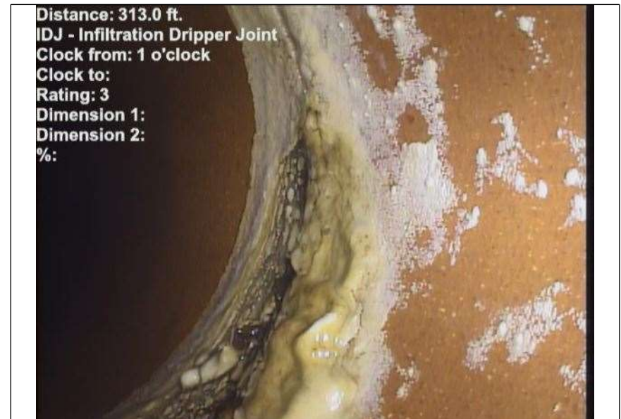
At: 313 ft. 1/. IDJ - Infiltration Dripper Joint Joint: Yes
