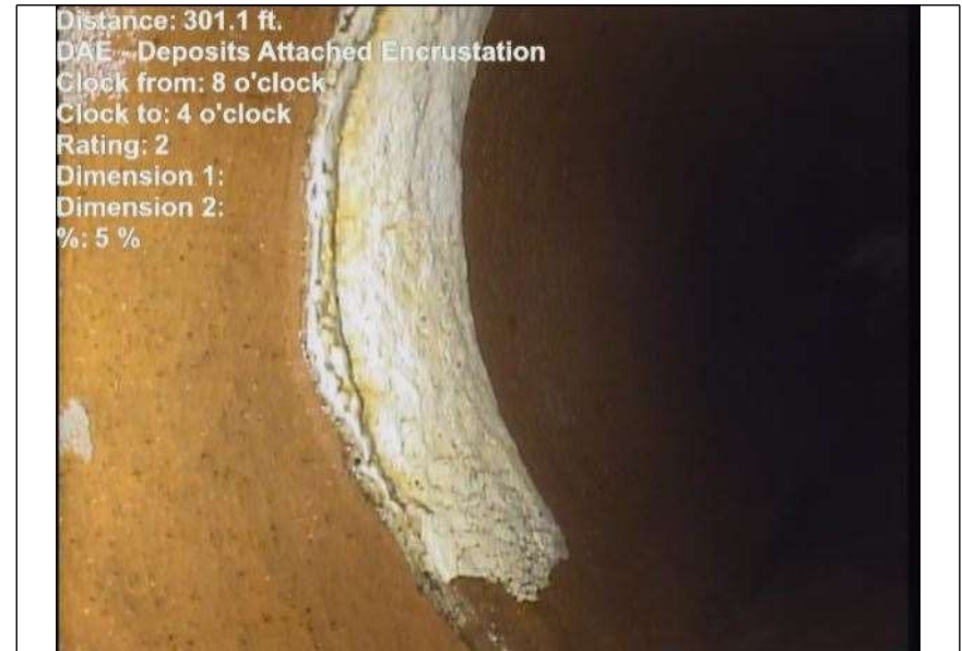
At: 301.1 ft. 8/4 DAE - Deposits Attached Encrustation Joint: No 5 %
