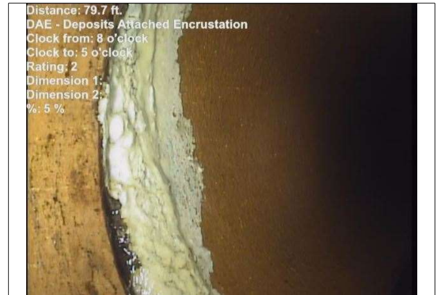
At: 79.7 ft. 8/5 DAE - Deposits Attached Encrustation Joint: No 5 %
