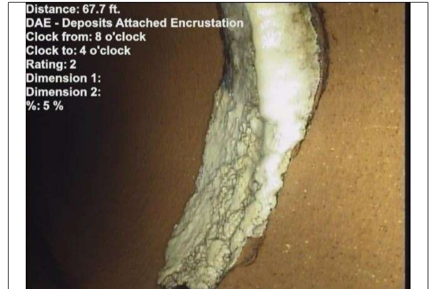
At: 67.7 ft. 8/4 DAE - Deposits Attached Encrustation Joint: No 5 %
