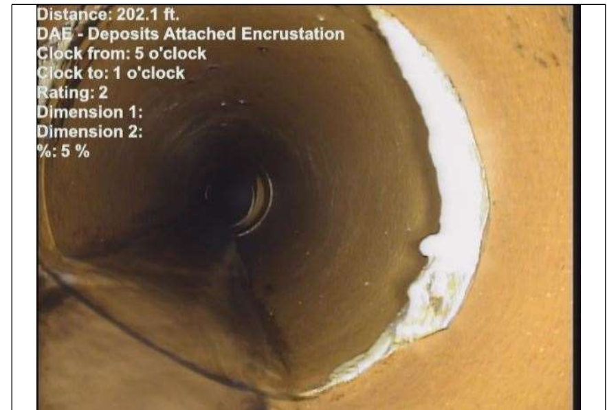
At: 202.1 ft. 5/1 DAE - Deposits Attached Encrustation Joint: No 5 %
