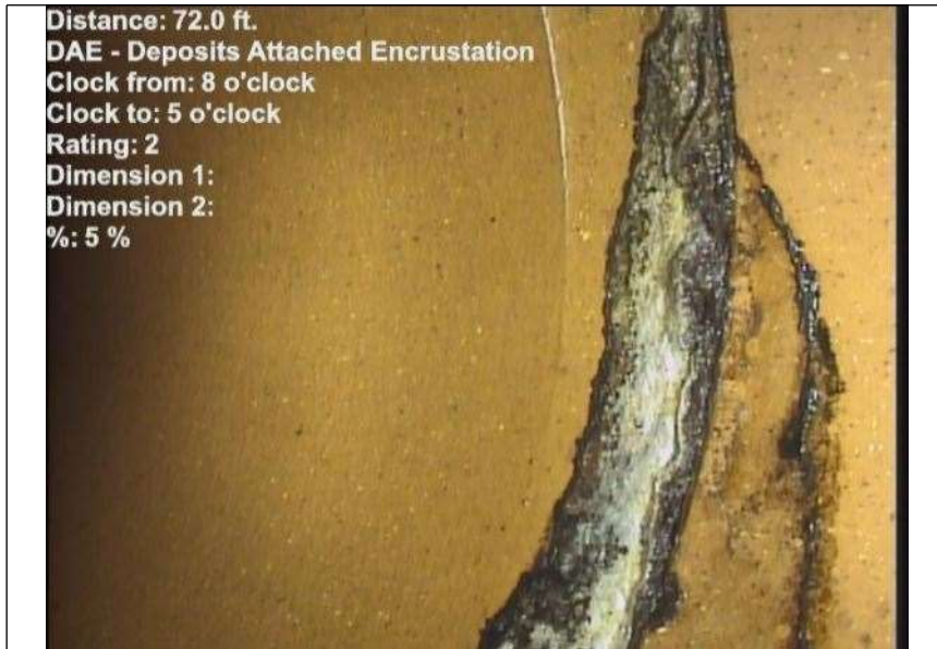
At: 72 ft. 8/5 DAE - Deposits Attached Encrustation Joint: No 5 %
