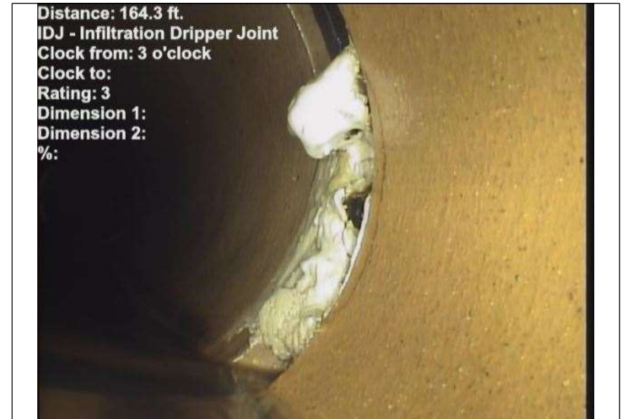
At: 164.3 ft. 3/. IDJ - Infiltration Dripper Joint
