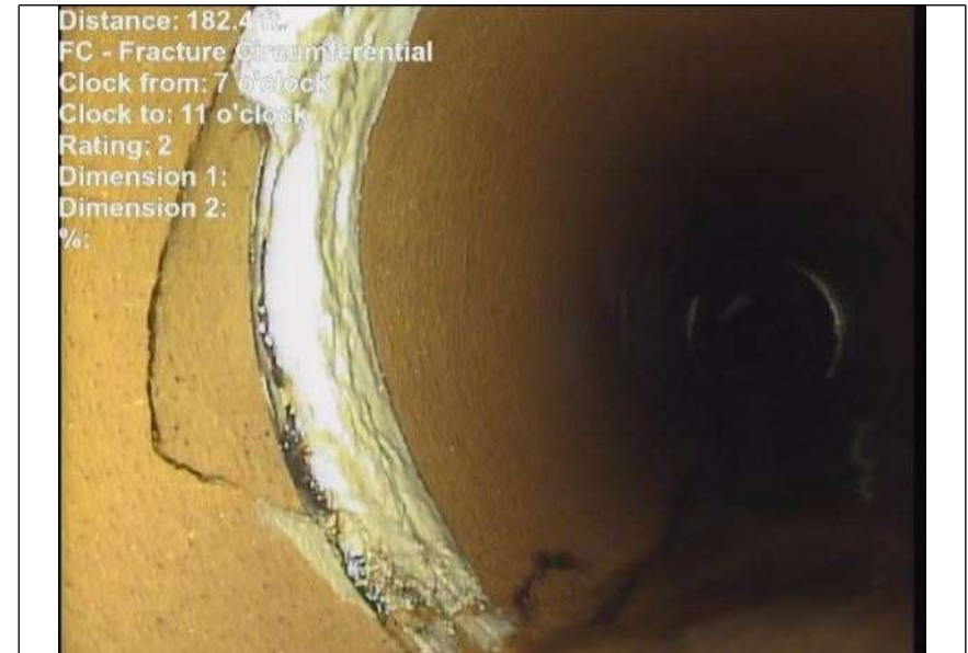
At: 182.4 ft. FC - Fracture Circumferential 7/11 Joint: No
