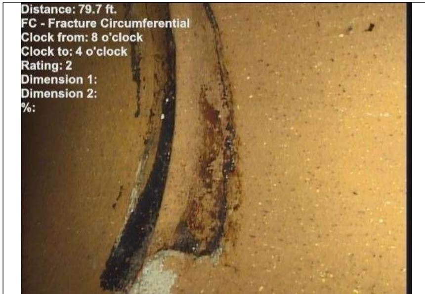
At: 79.7 ft. 8/4 FC - Fracture Circumferential Joint: No
