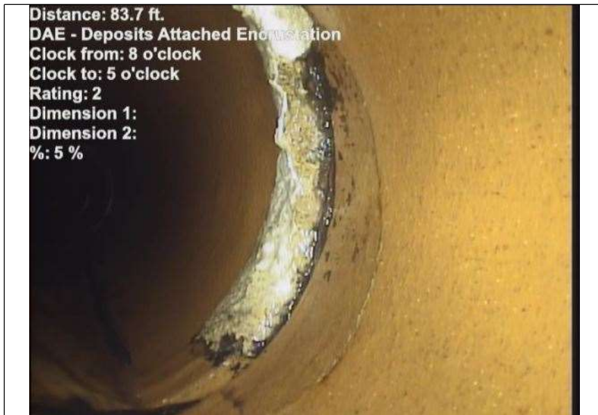
At: 83.7 ft. 8/5 DAE - Deposits Attached Encrustation Joint: No 5 %
