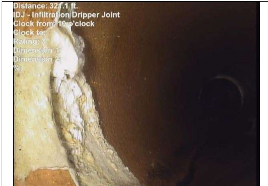
At: 321.1 ft. 10/ IDJ - Infiltration Dripper Joint Joint: Yes
