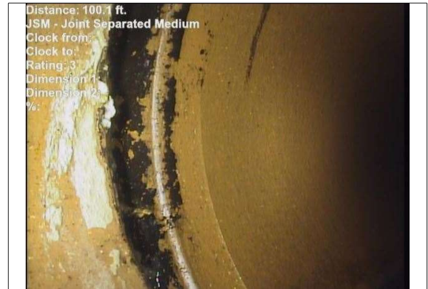
At: 100.1 ft. JSM - Joint Separated Medium Joint: No
