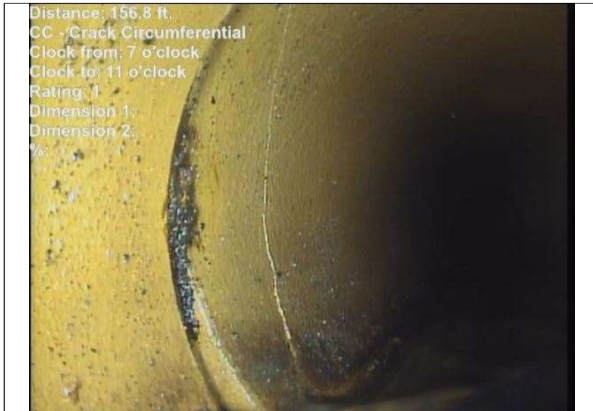
At: 156.8 ft. CC - Crack Circumferential 7/11
