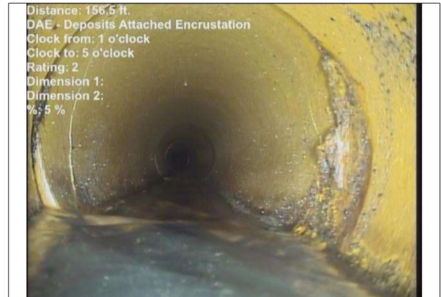
At: 156.5 ft. 1/5 DAE - Deposits Attached Encrustation Joint: No 5 %
