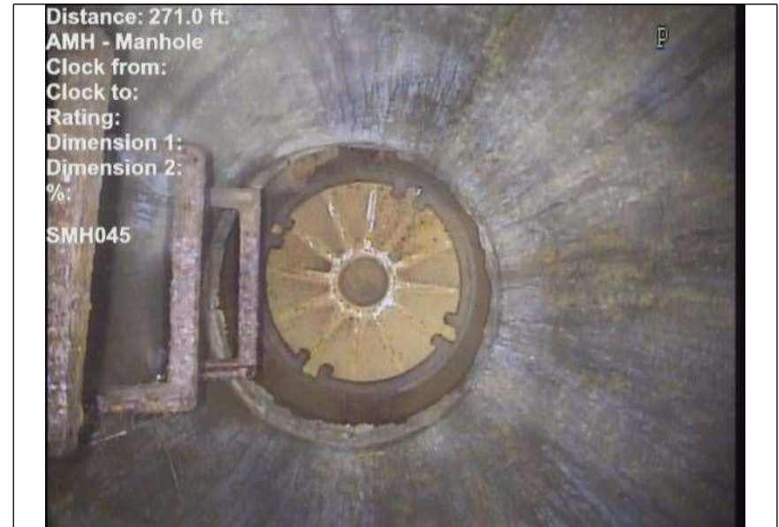
At: 271.1 ft. AMH - Manhole Joint: No SMH045
