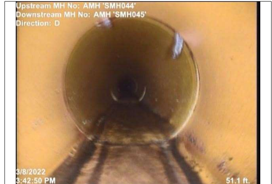
At: 53 ft. 11/2 DAE - Deposits Attached Encrustation Joint: No 5%
