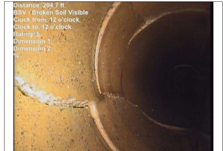
At: 204.7 ft. 12/12 BSV - Broken Soil Visible Joint: No
