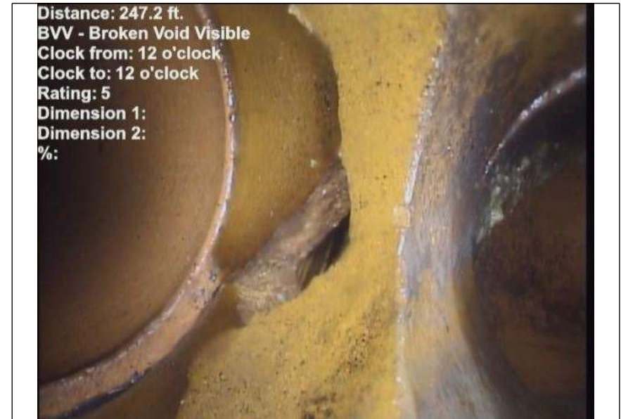
At: 247.2 ft. BVV - Broken Void Visible 12/12 Joint: No
