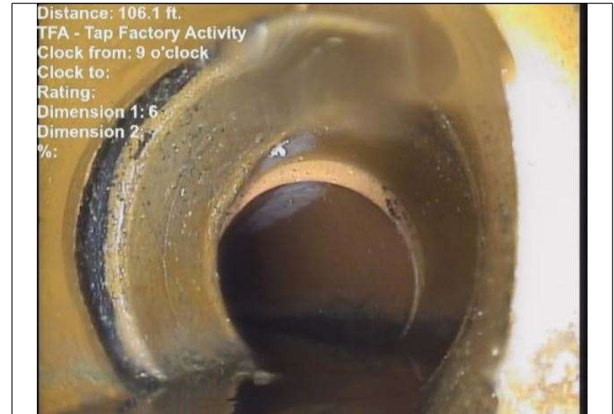
At: 106.1 ft. 9/. TFA - Tap Factory Activity Joint: No
