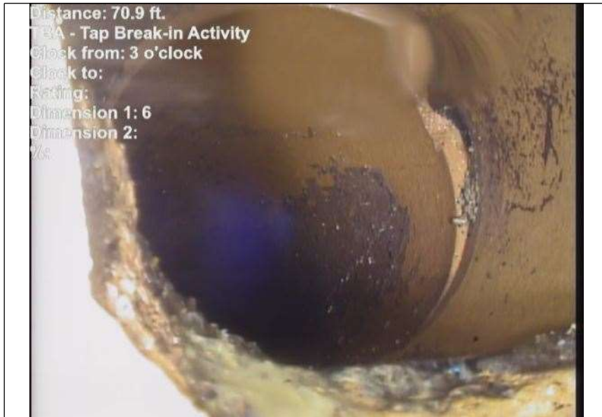
At: 70.9 ft. 3/. TBA - Tap Break-in Activity Joint: No
