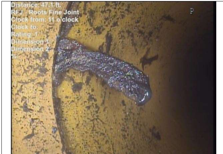
At: 47.1 ft. 11/. RFJ - Roots Fine Joint Joint: Yes
