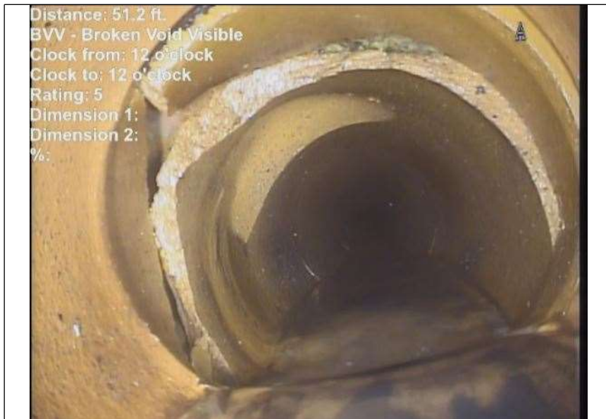
At: 51.2 ft. BVV - Broken Void Visible 12/12 Joint: No
