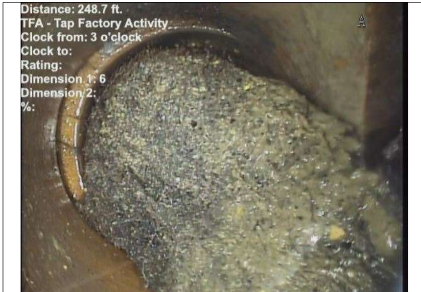
At: 248.7 ft. 3/. TFD - Tap Factory Defective Joint: No RTL
