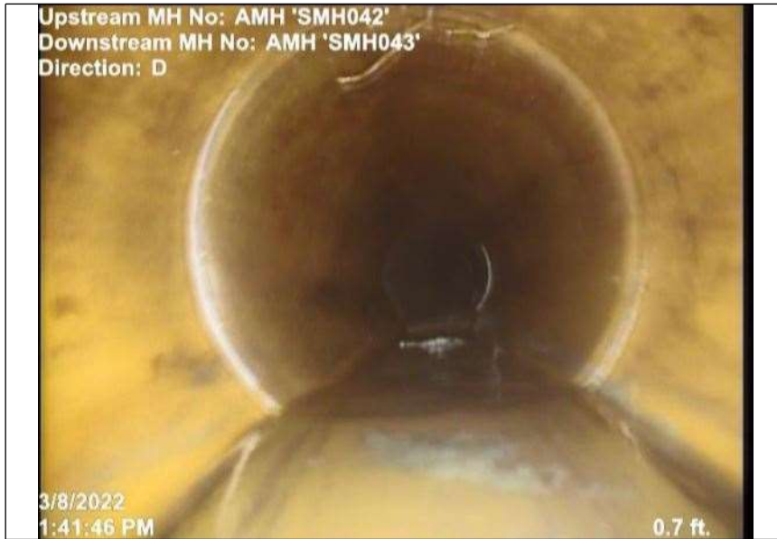
At: 0.994 ft. RFJ - Roots Fine Joint 12/1 Joint: Yes
