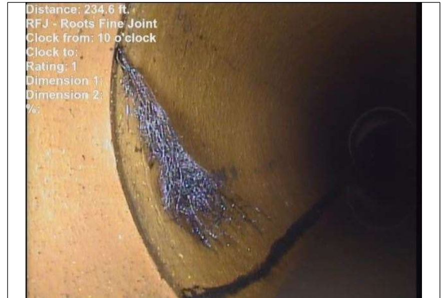
At: 234.6 ft. 10/. RFJ - Roots Fine Joint Joint: Yes
