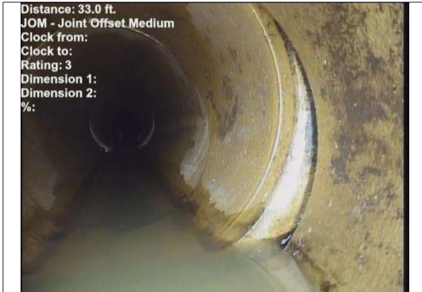
At: 33 ft. JOM - Joint Offset Medium Joint: No
