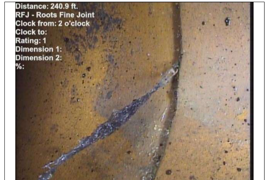
At: 240.9 ft. 2/. RFJ - Roots Fine Joint Joint: Yes
