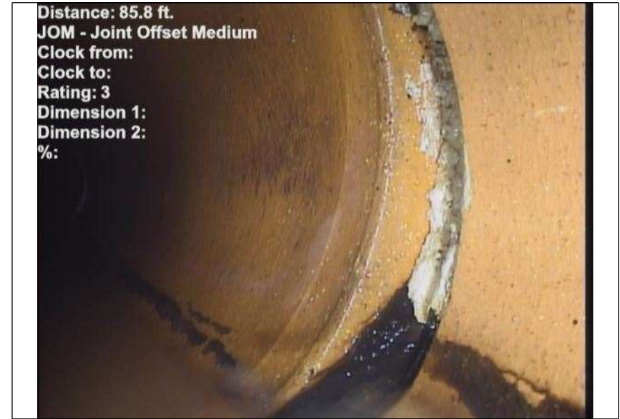
At: 85.8 ft. JOM - Joint Offset Medium Joint: No
