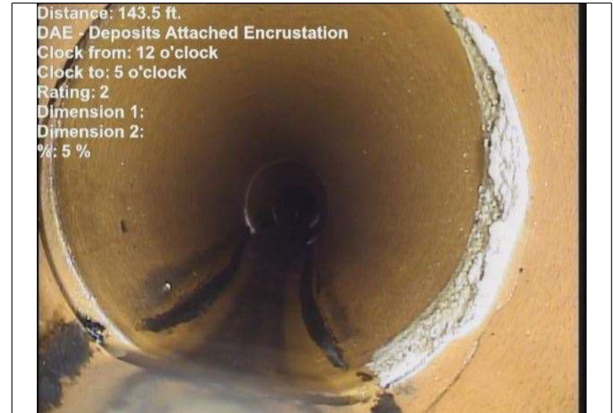
At: 143.5 ft. DAE - Deposits Attached Encrustation 12/5 Joint: No 5 %
