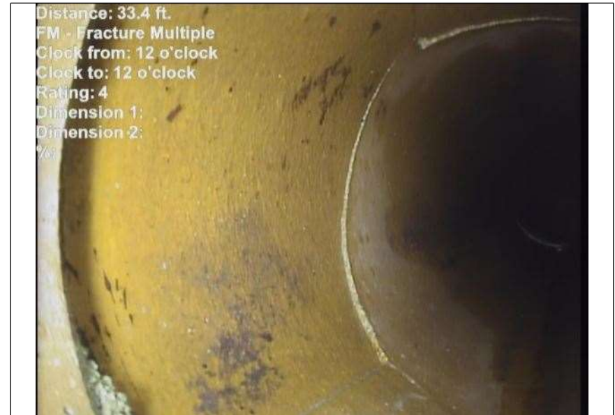
At: 33.4 ft. 7/5 FM - Fracture Multiple Joint: No
