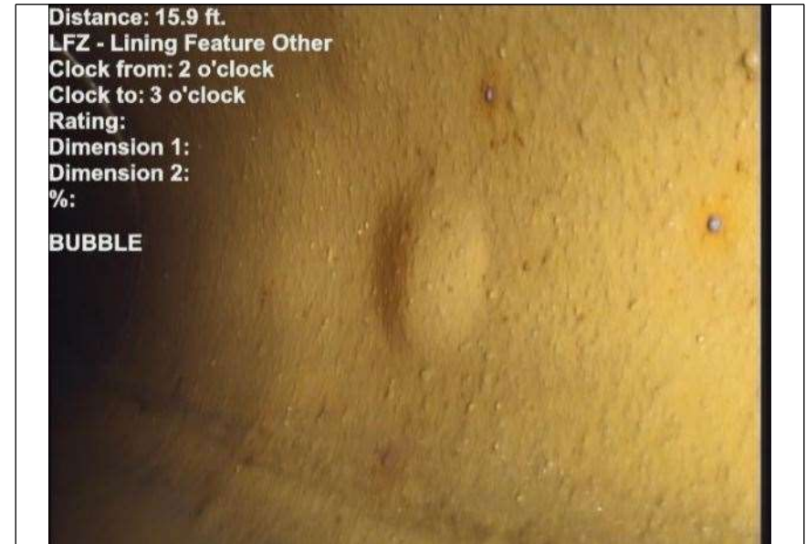
At: 15.9 ft. 2/3 LFZ - Lining Feature Other Joint: No BUBBLE
