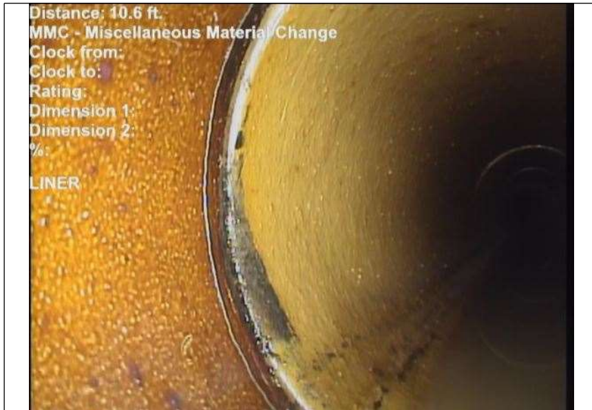
At: 10.6 ft. RPR - Point Repair Replacement Joint: No LINER
