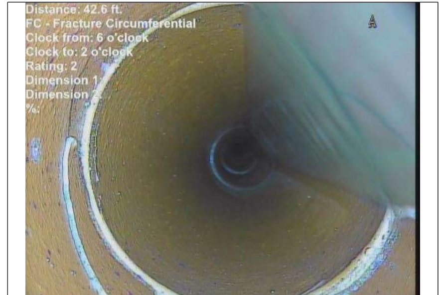
At: 42.6 ft. 6/2 FC - Fracture Circumferential Joint: No
