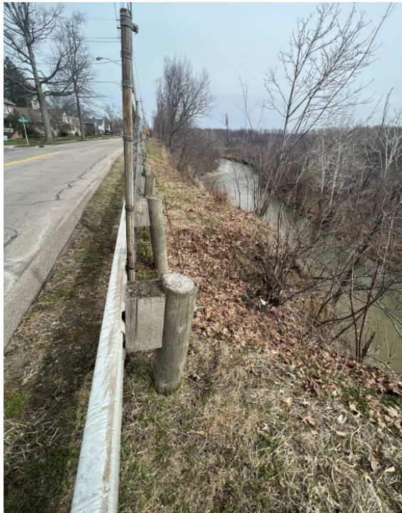
Photo 4: Depicting the magnitude of the slope looking north along River Street.
