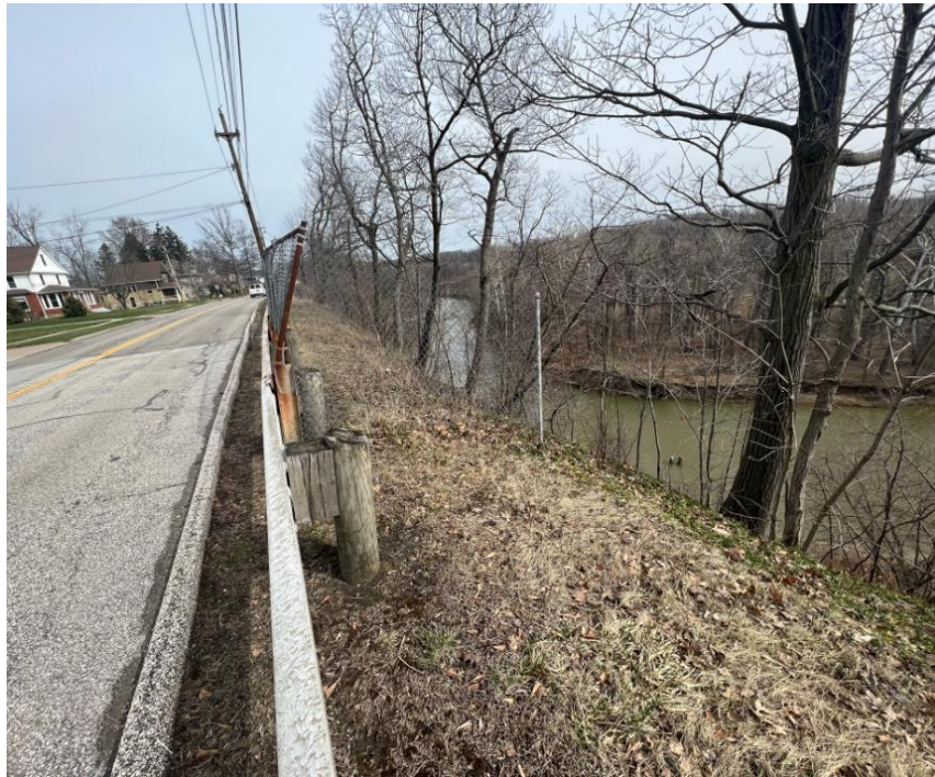
Photo 2: Depicting the general site conditions at the crest; looking north along River Street.
