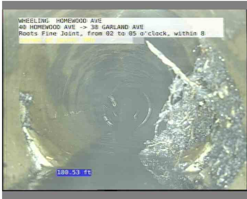
13, 00:14:30, 180.53ft Roots Fine Joint, from 02 to 05 o'clock, within 8 inches of joint: YES
