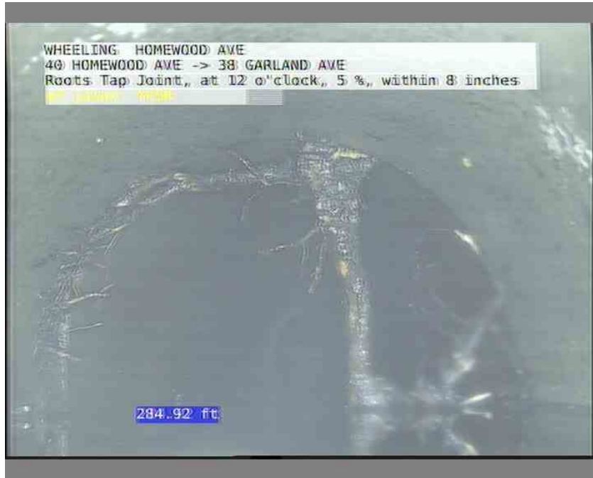
19, 00:24:28, 284.92ft Roots Tap Joint, at 12 o'clock, 5 %, within 8 inches of joint: YESR
