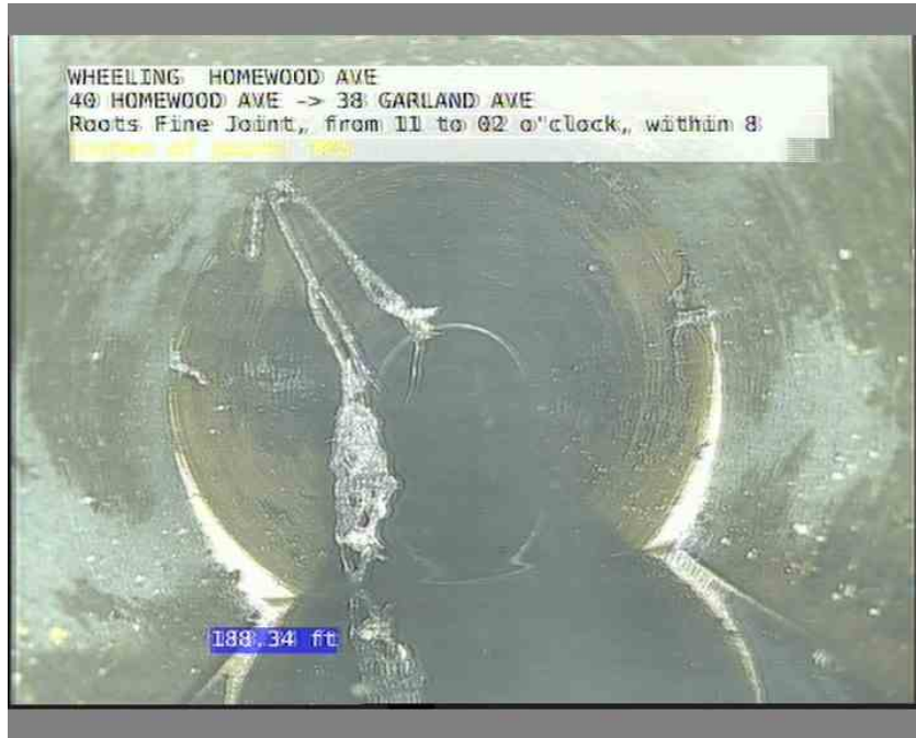
15, 00:15:48, 188.34ft Roots Fine Joint, from 11 to 02 o'clock, within 8 inches of joint: YES
