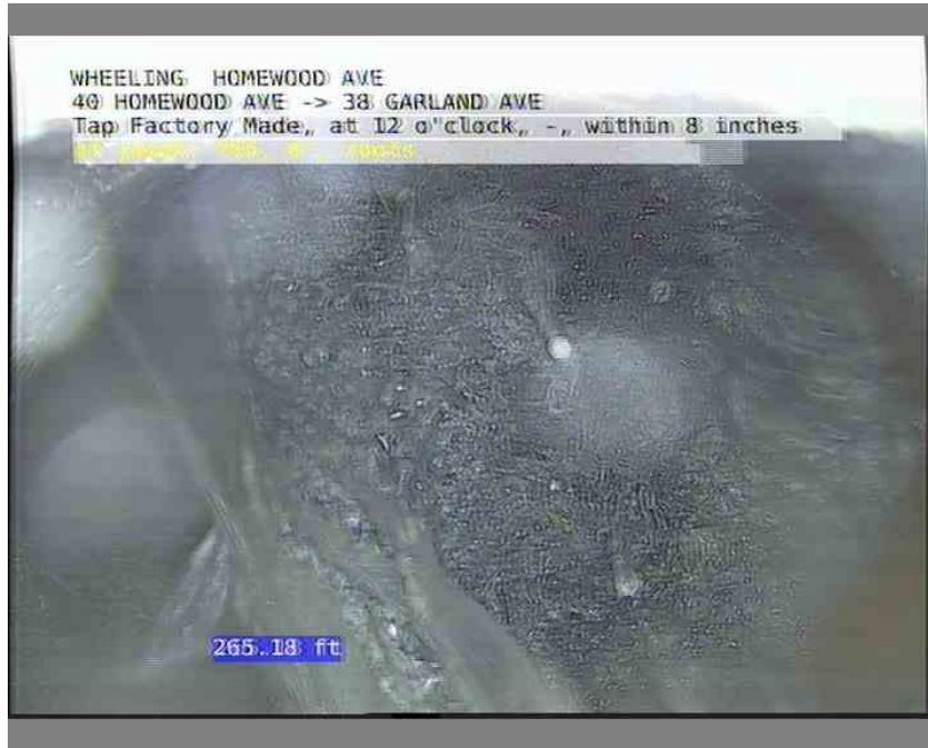
17, 00:20:42, 265.18ft Tap Factory Made, at 12 o'clock, -, within 8 inches of joint: YES, 6" / roots
