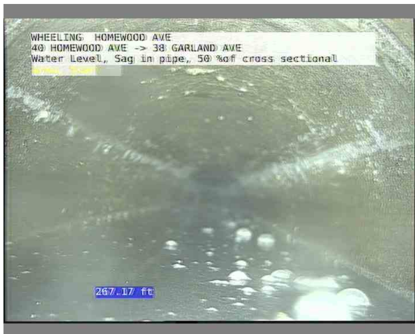
18, 00:21:24, 267.17ft Water Level, Sag in pipe, 50 %of cross sectional area, Start
